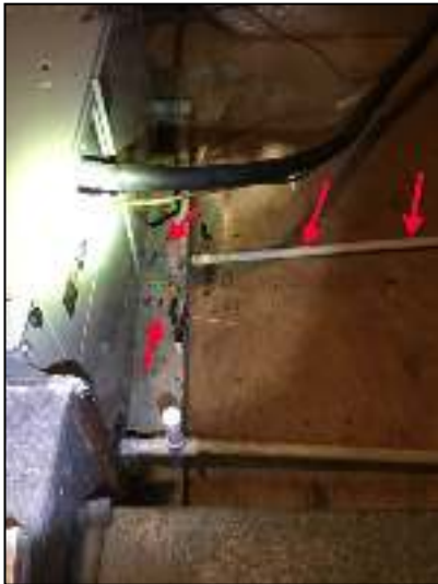
Repair drain pipe from heat pump in attic to flow properly. Clean pan area.
