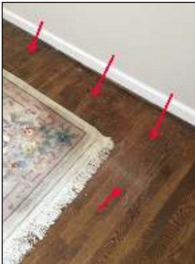
Repair hard wood flooring at top back right bedroom under windows.
