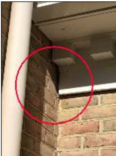
Seal opening at brick to lower eave area front left of garage to house corner.
