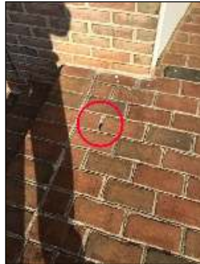
Repair brick joint at left of front entrance.
