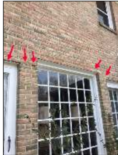
Repair brick joints above back door and window corners.
