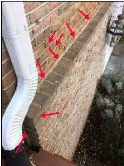
Repair crack at top edge area of brick to lower level. Left end.
