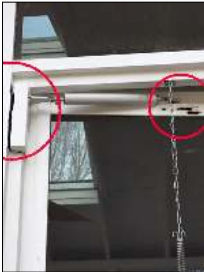
Replace back enclosed porch door and trim area that is rotted.
