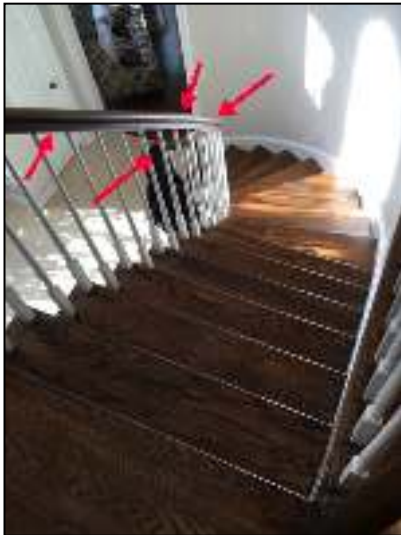
Secure hand rail at outside edge railing on main steps.
