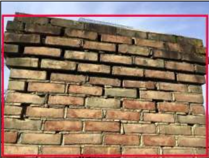
Repair all deteriorated mortar joints on both chimneys at top 4ft of bricks
