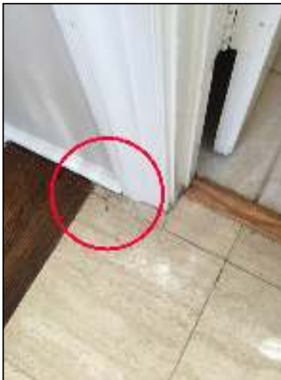
Repair tiles from main hall to kitchen left of door.
