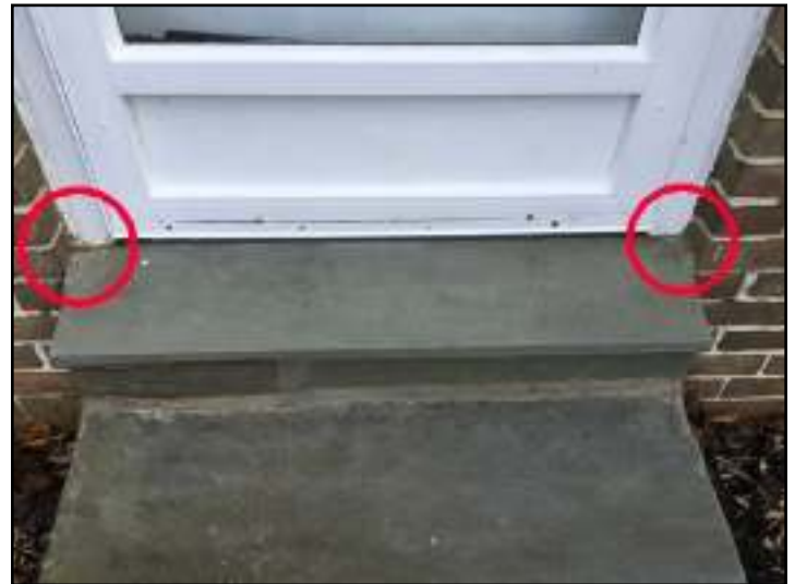
Seal sides of back center door step stone areas several locations.
