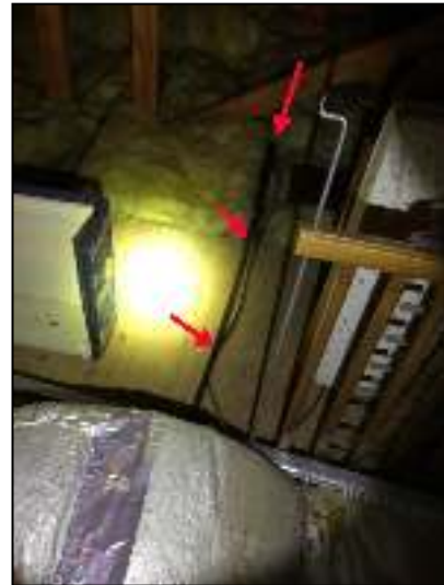
Remove abandoned refrigerant lines behind attic unit through floor to basement from attic.
