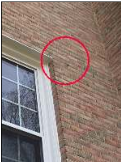
Repair brick joint left end above right side of second level window.
