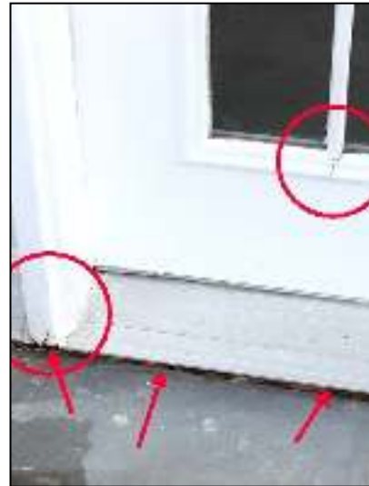
Replace rotted wood trim around left end lower level door and repair or replace damaged door. Caulk brick to trim areas.
