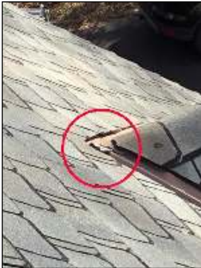
Seal metal terminations at top edges of dormers on front garage area.
