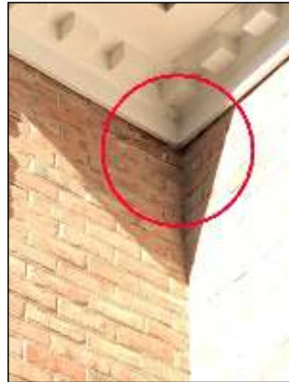
Repair brick joints at right side of front porch at eave and seal opening.
