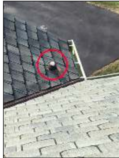
Extend front left plumbing vent on roof to 10" minimum.
