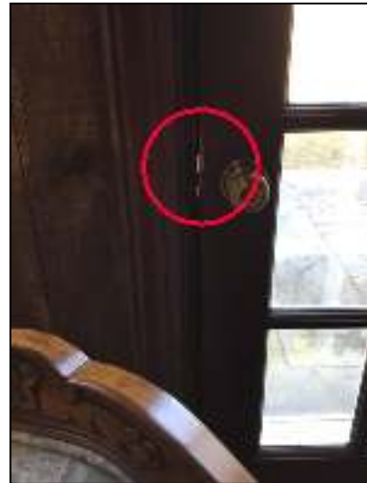
Provide tight seal around all back main level single doors to exterior.
