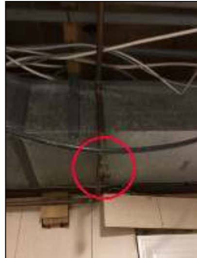
Replace leaking plumbing cap above main electric panels.
