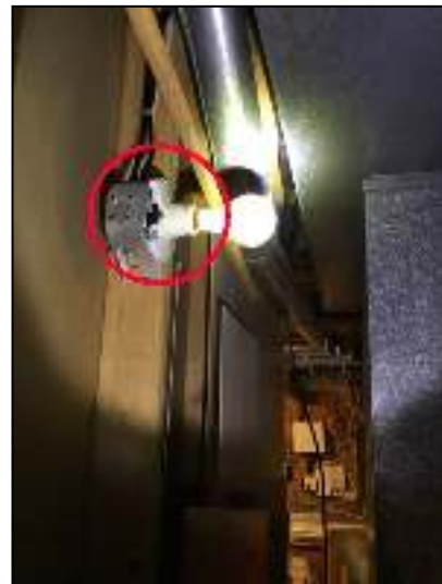
Replace damaged fixture and install globe on bulb behind basement furnace area.
