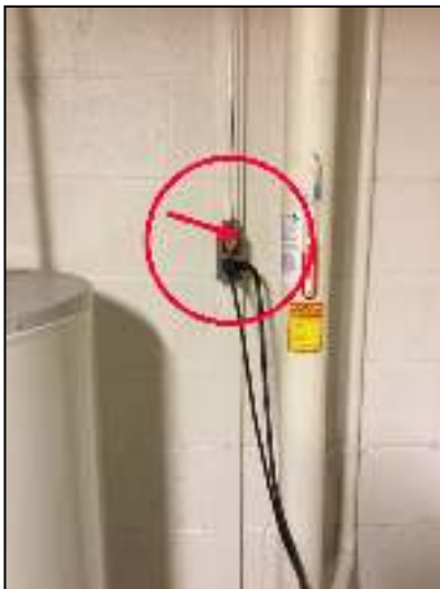
Eliminate orange extension cord on outlet at sump pump by water heater.
