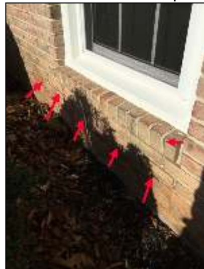
Repair large open brick joint on front of garage wall under front left window and above right front garage window. Right corner of window.
