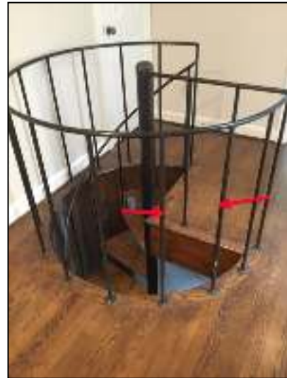
Provide no more than 4" openings in railings on spiral stairs. Child fall safety issue.
