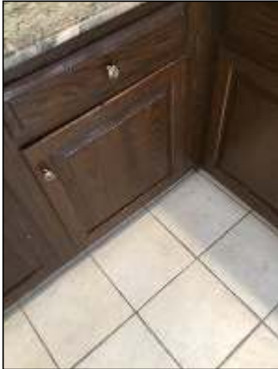
Repair hardware on several kitchen cabinets.
