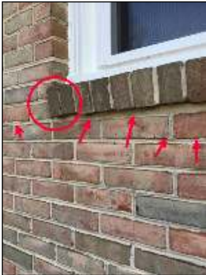
Repair brick joints at back top left single window area. And at top right corner of same window.
