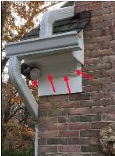
Replace rotted wood at right side back corner.
