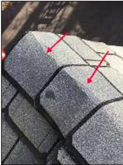
Replace damaged cap shingles right end of house on top peak end
