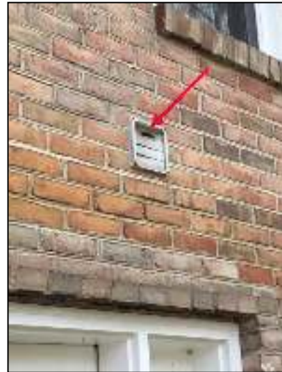
Replace damaged vent cover at left end wall
