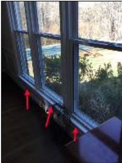
Several front and back main level windows are lower than 18" safety limit and need to be safety glass rated.
