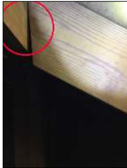
Properly secure all hip roof rafter ends right end of attic at rafter ends. Several terminations. .
