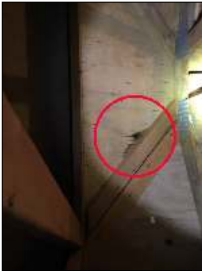
Repair minor roof leak at right of attic air handler, right top peak area.
