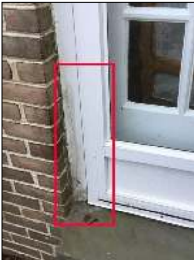
Replace rotted trim at back right single door
