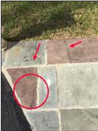
Repair cracked stone at front entrance. Left side.
