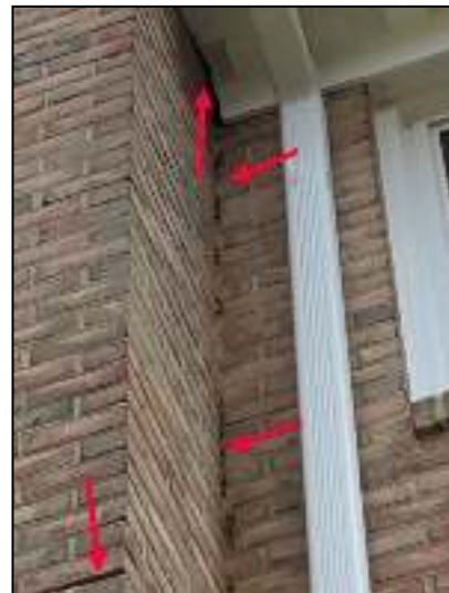
Seal gap at left end chimney to house area and at soffit this area. Repair brick joints at left chimney base cap area left end. seal opening at soffit ara.
