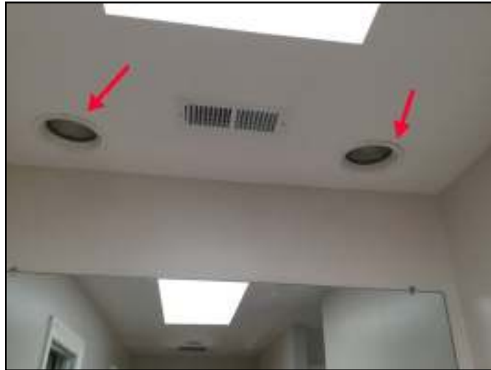
Secure recessed lighting in Master bedroom at makeup desk area.
