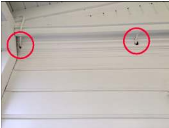
Seal openings at wires above back porch enclosure house end.
