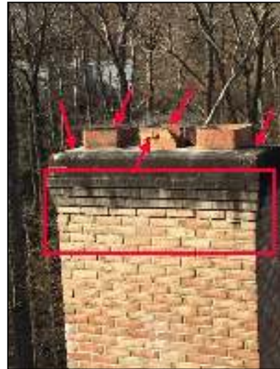
Replace damaged flue and top cap screening on left chimney. Also repair mortar joints around top 4ft section. Repair both chimney top cap concrete.
