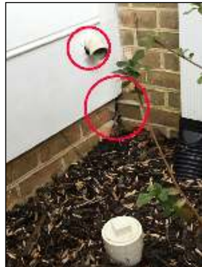
Seal openings at back right of porch enclosure at house to porch area and around piping.
