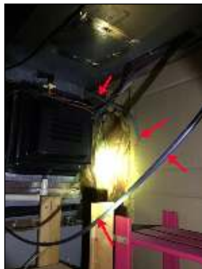
Remove all abandoned electric wiring behind furnace area and at left of main panels
