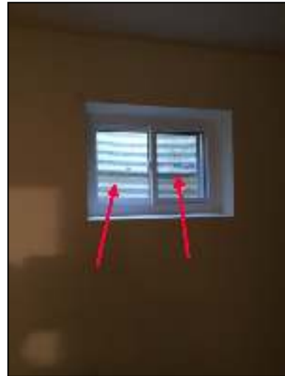
Basement rooms cannot be used as bedrooms unless they have the required size egress windows and exterior clearance. Fire safety.
