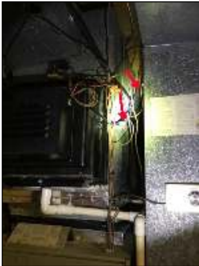
Install outlet for humidifier to eliminate extension cord.
